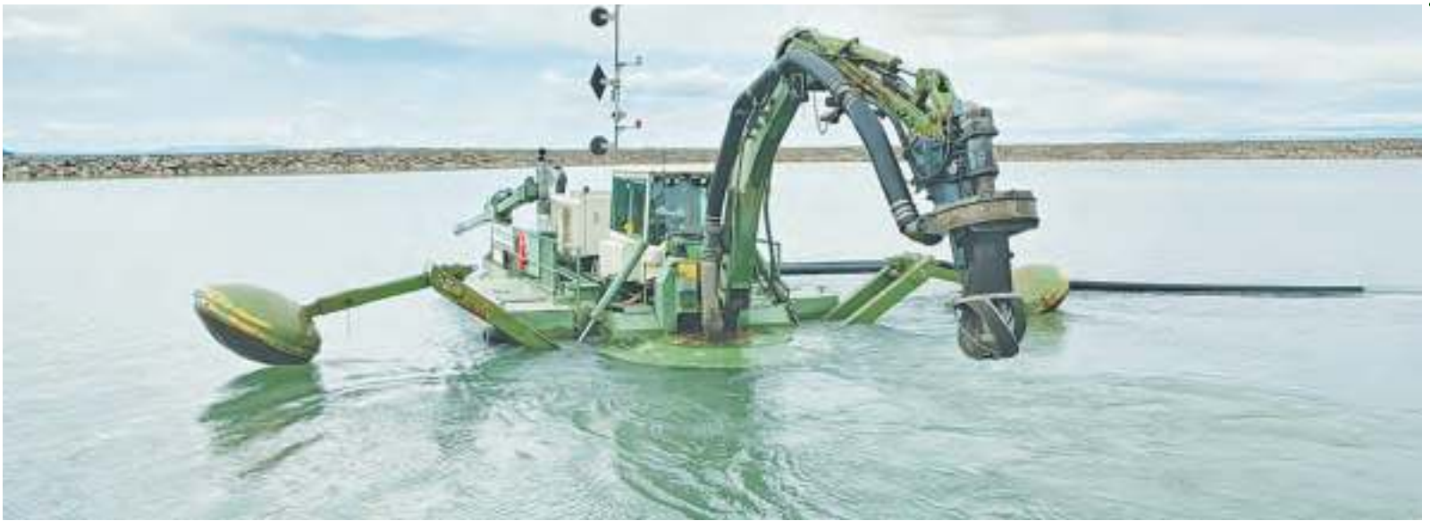
WATERMASTER amphibious dredger increases the depth of the newly-constructed Karema Port on Lake Tanganyika in Katavi Region.
